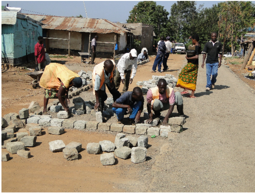
Laying of a stone block foundation in preparation for the laying of a concrete mix at Uhanya beach
