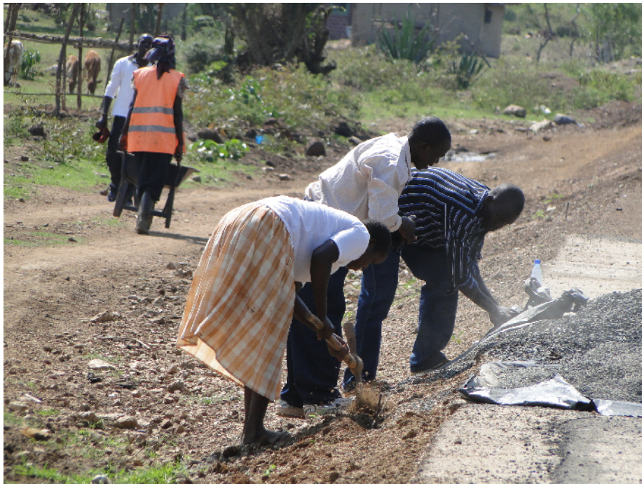
Finishing of the road shoulders is ongoing as the laying of a low-seal progresses towards Nyenye
