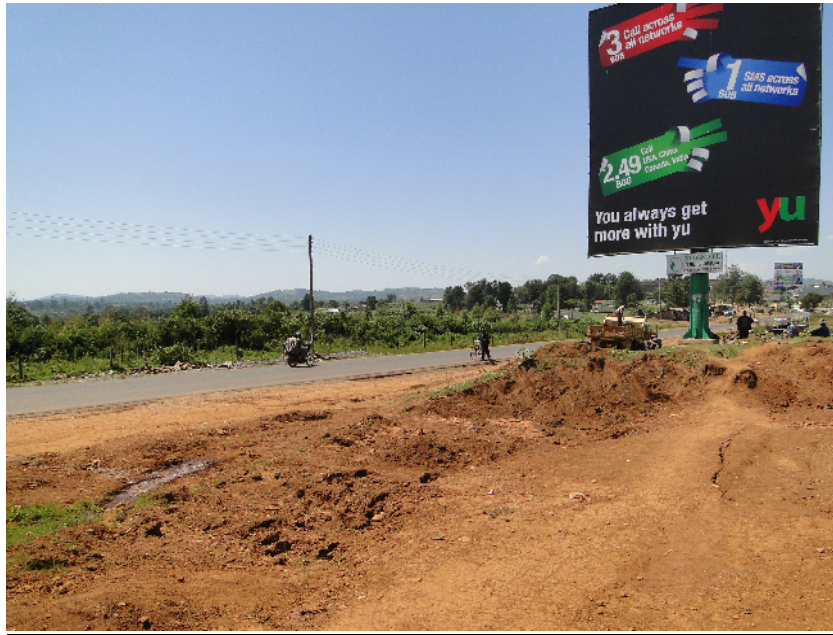
4.1. At the junction with Kisii-Sotik(B3) road, where a parking bay is to be constructed, site clearance is taking place
