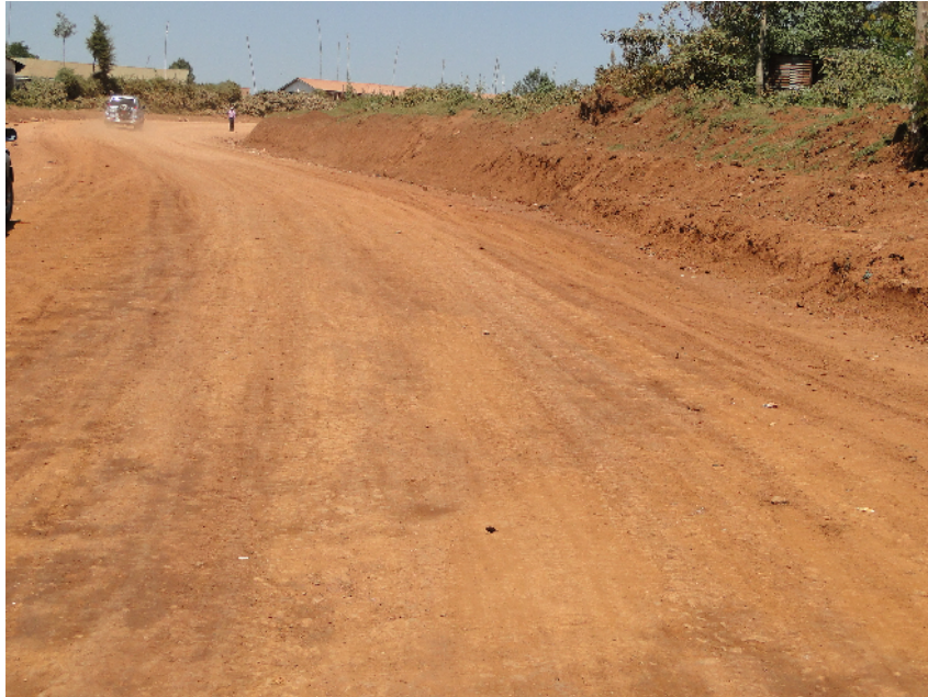
4.2. Earthworks and laying of the subbase material has been done upto km3.5
